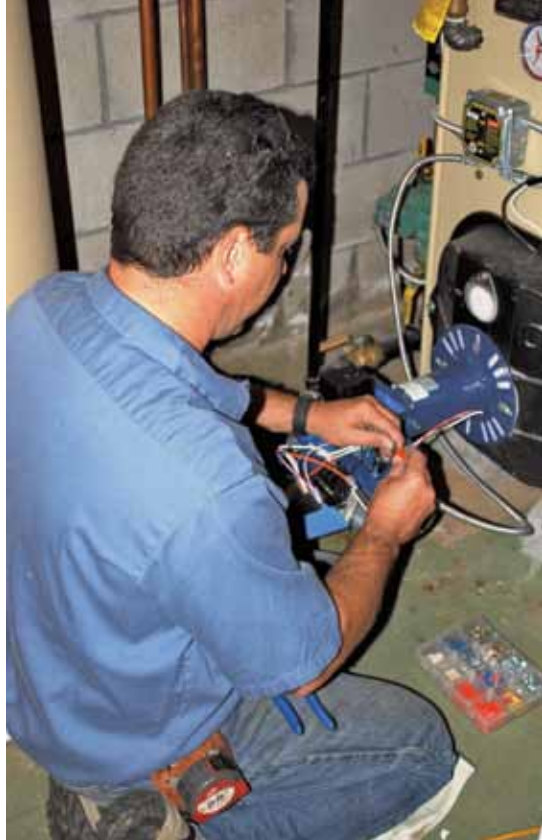
Russ St. Gelais, a service technician for Vermont Gas, works on a conversion project. Today, 62 percent of the homes and businesses in the new communities that had been using heating oil or propane use natural gas.
